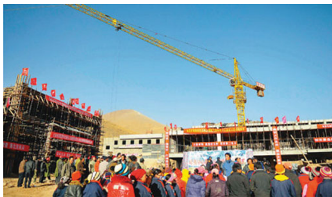
Figure 8. Roof-sealing for a primary school building with the highest altitude in the disaster area (under the partner assistance of Beijing Municipality)
