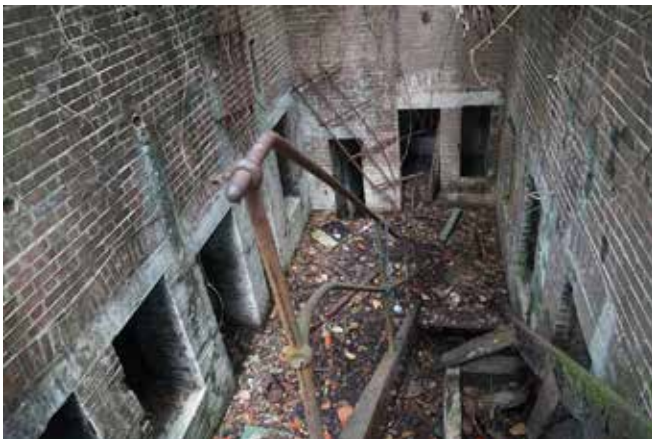
The first step is a long one! This is the Serapong Spur 9.2 in shell store and magazines, which were converted for the use of the 6 in Emplacement No. 1 in 1937.
